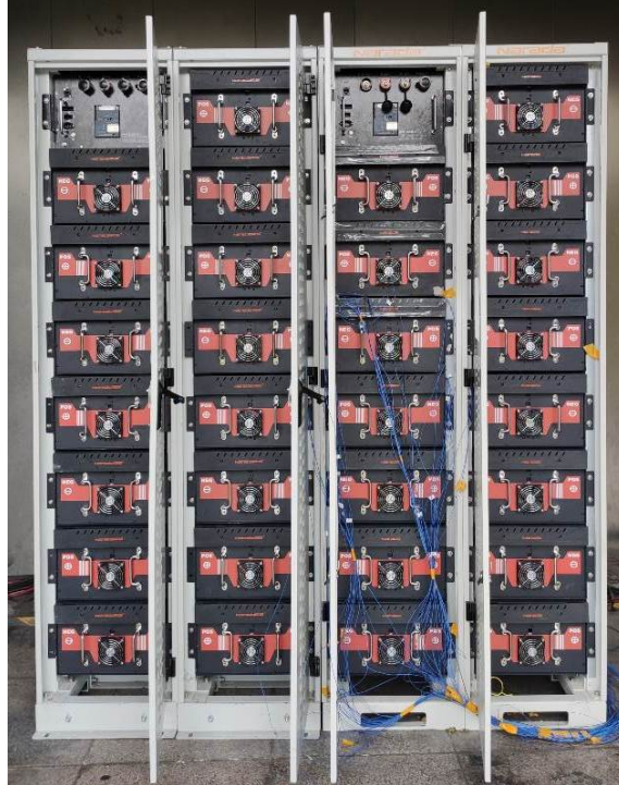
Overview – Unit after test
